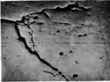
NO. 41. SHOWING SLAG CRACKS.
